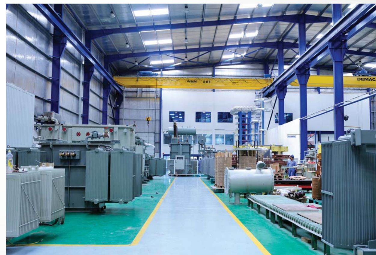
Inside view of the plant (assembly section)
