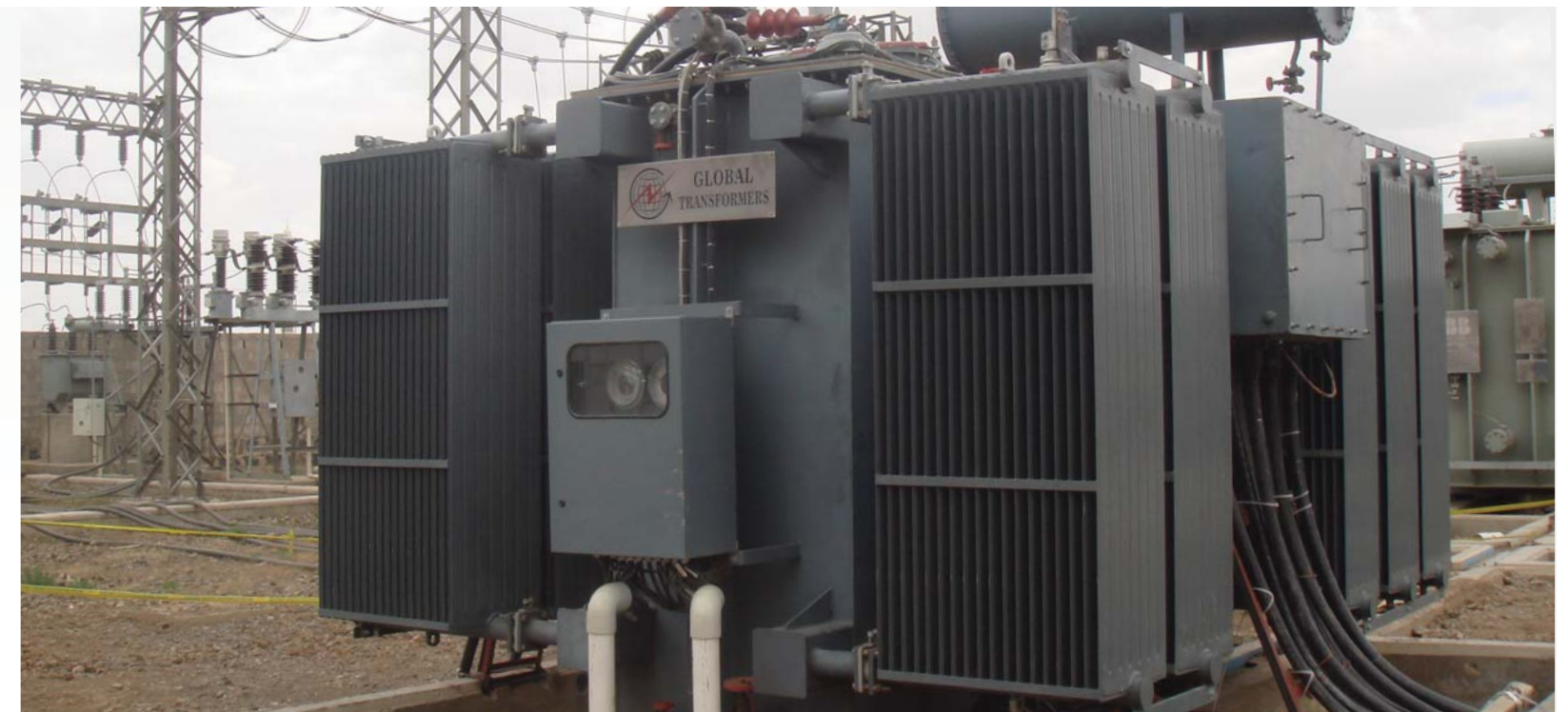
Commissioned at Site (Yemen)
