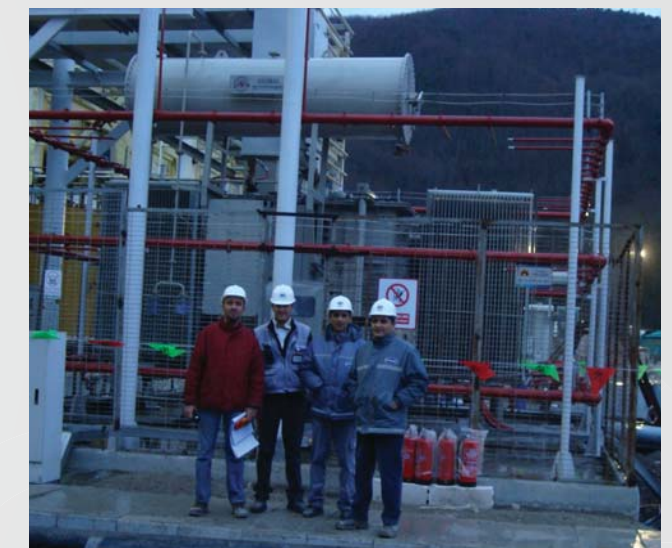
63MVA, 33KV/6.3-6KV Commissioned at Site (Turkey)
